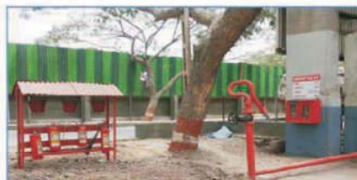
Proper Fire Hydrant System
