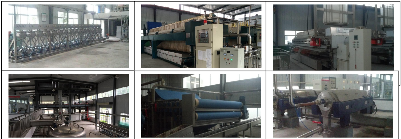
Note: new equipment installed at the plant
