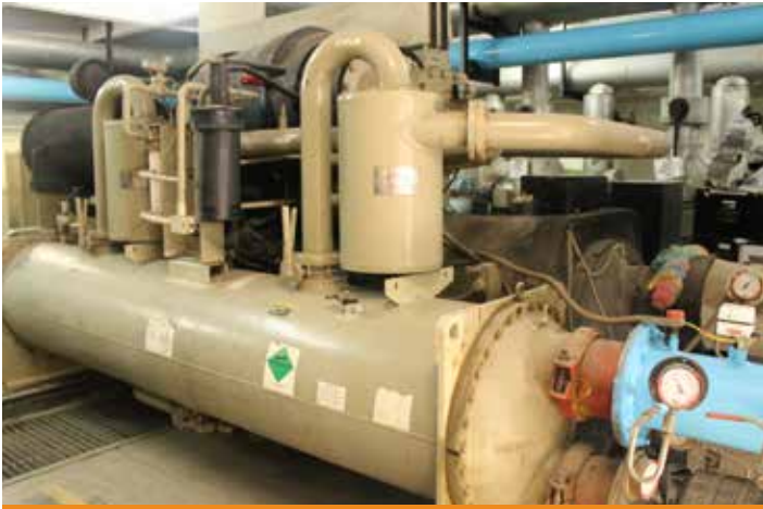
RETROFITTED CHILLER SYSTEM, MAHINDRA TOWERS.
