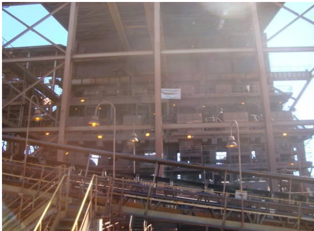
Figure 2: Before Cleaner Production : lamps lighted during the daytime period
